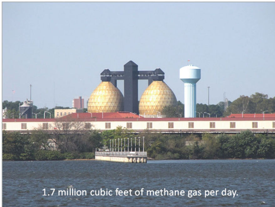
Fig. 18.11 Anaerobic digesters of the Back River wastewater treatment plant in Baltimore, MD. On-site renewable electricity generation of high-efficiency, gas turbine generators produces 3 MW continuously plus heat for these thermophilic digesters. This reduces the energy-related operating cost an average of $1.4 million annually, according to Baltimore City Dept. of Public Works. This industrial process can be enhanced using electromethanogenesis. (Photo by Mark Jonas)
