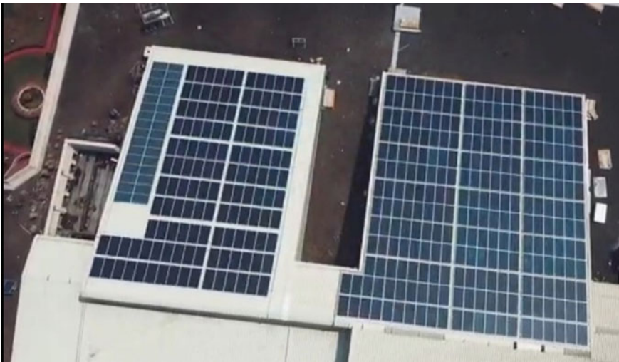
Fig. 3 The grid-tied PV array
