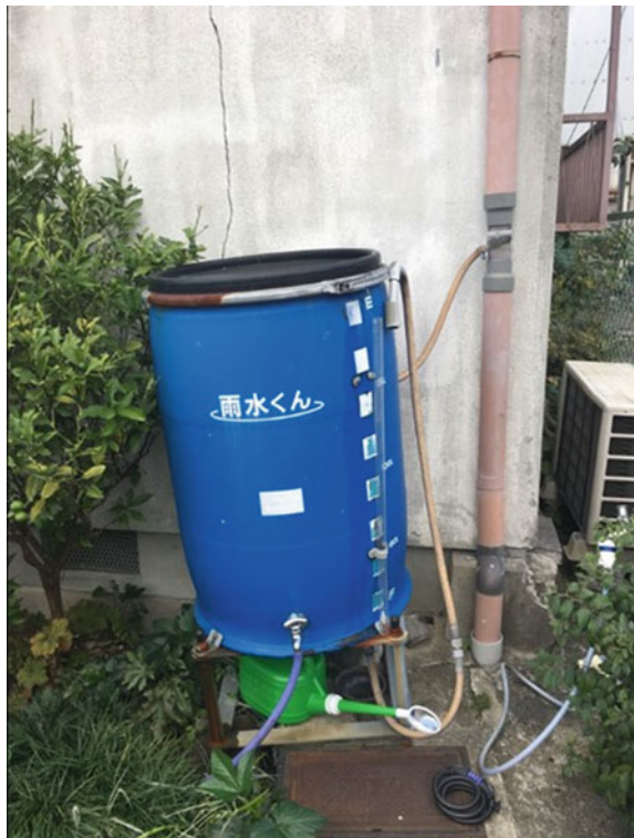
Photo 14.5 Rain water tank
