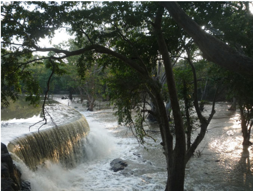
Fig. 19.2 Tekkam Barrage at Malwathu River, Mannar ( Photo credit Eng. Badra Kamaladasa)
