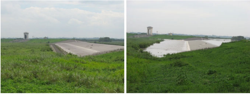
Fig. 20.11 The overflow levee in the third regulating pond. Each picture is a view from the north, and the Watarase River flows on the right side of the levee. The photo on the right shows overflow from the river on September 7, 2007
