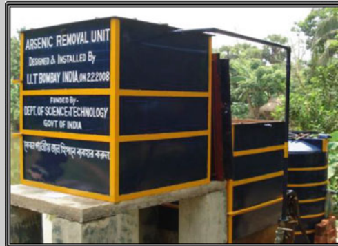
Fig. 9.7 IIT Bombay developed arsenic removal units
