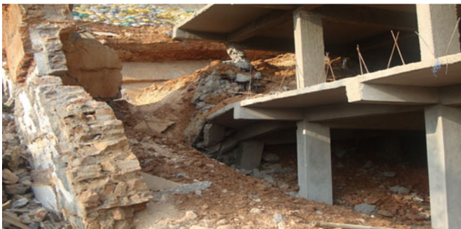
b) Damaged apartment in construction due to retaining wall collapse
