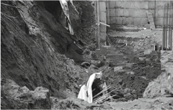
Fig. 3 Deep excavation failure in clayey silty sand at a construction site in Visakhapatnam
