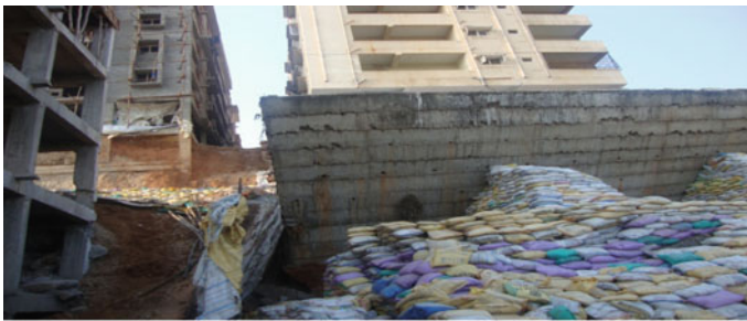
a) View of failed retaining wall
