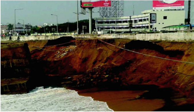
Fig. 4 Eroded beach affecting neighbouring footpath at Visakhapatnam
