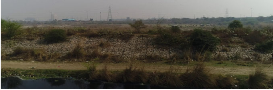
Fig. 22 Guide bund protection at Delhi Noida bridge after 20 years
