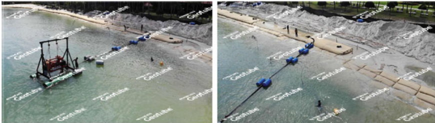
Fig. 26 The sand was hydraulically pumped from the shallow waters direct into the geotextile tube
