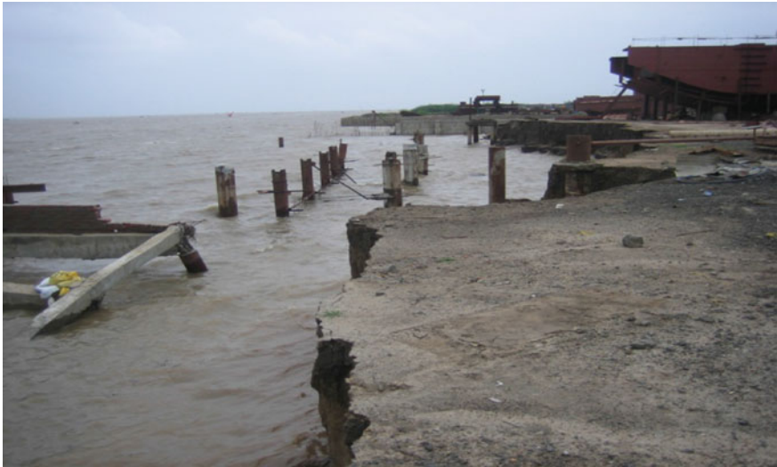
Fig. 3 Critical state of erosion—note state of earlier control measures
