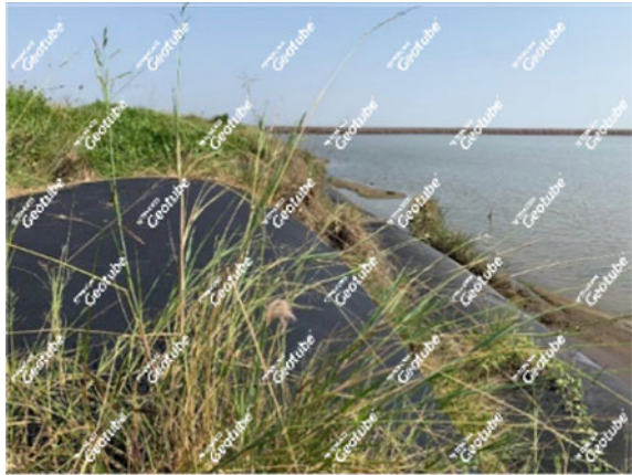
Fig. 17 Vegetation growth over the sand filled mattress and geotextile tube
