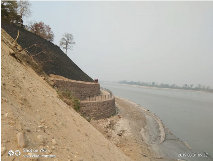
Fig. 25 Reinforced soil wall, launching apron, and erosion control mat at Valmiki Nagar
