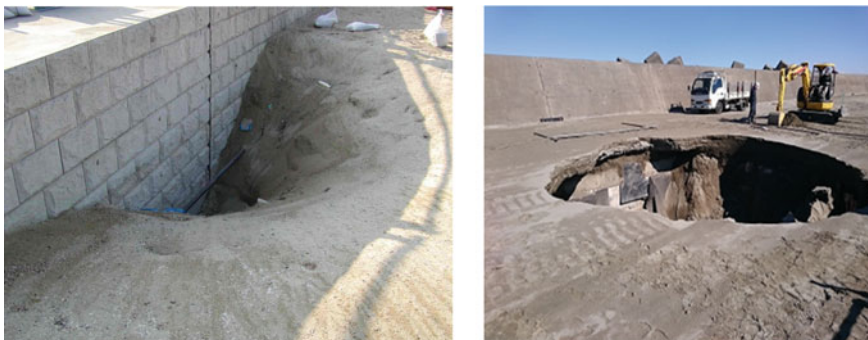
Fig. 8 Cavity collapses behind seawalls
