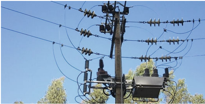
Fig. 3 Structural view of the transmission lines of the transformer
