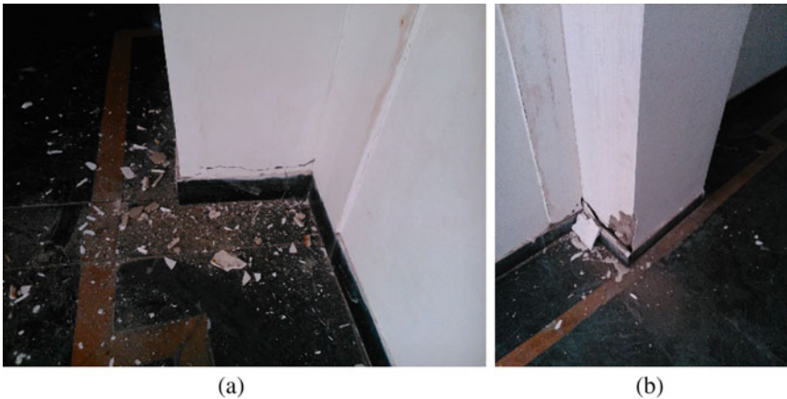
Fig. 1 Columns (fourth level) of Royal Group of Institution in Guwahati that faced damages due to the Imphal earthquake 2016
