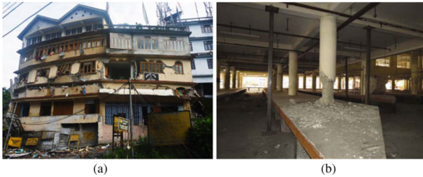
Fig. 4 a Total collapse at the second story leading to extensive damage at the third story of Moonlight School building at Chungthang, Sikkim [25], b Damages in the columns due to short column effect in the New Market building, Imphal [24]
