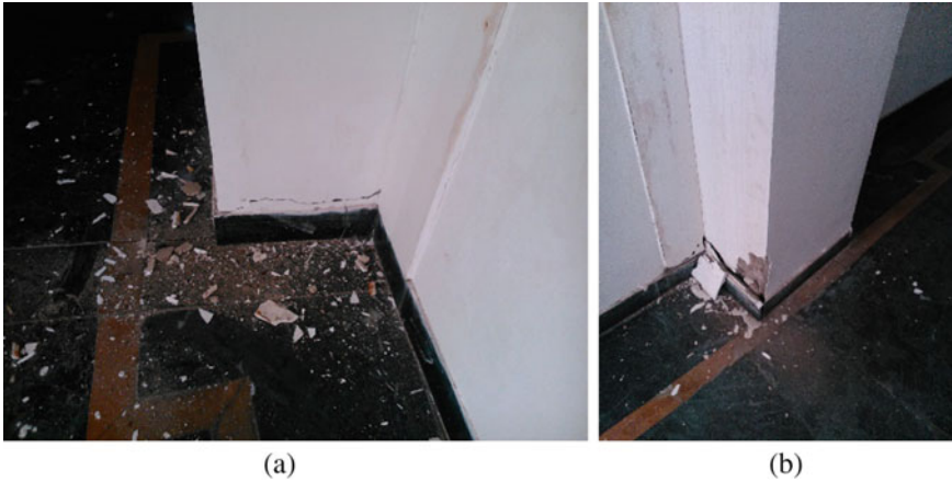
Fig. 1 Columns (fourth level) of Royal Group of Institution in Guwahati that faced damages due to the Imphal earthquake 2016
