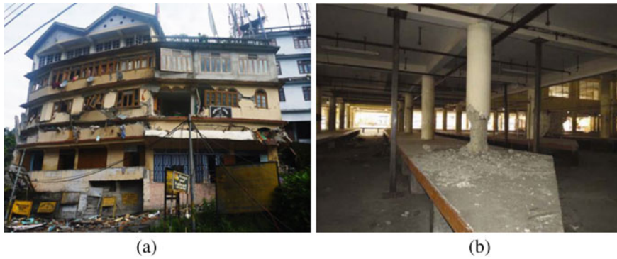
Fig. 4 a Total collapse at the second story leading to extensive damage at the third story of Moonlight School building at Chungthang, Sikkim [25], b Damages in the columns due to short column effect in the New Market building, Imphal [24]
