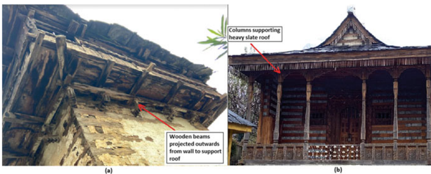
Fig. 7 a Cantilevered balcony in old Kath-kuni buildings. b Cantilevered balcony having columns to support the slate roof
