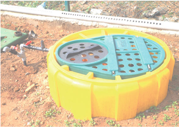
Fig. 18.4 Daphniafiltration unit at the Indian demonstration site
