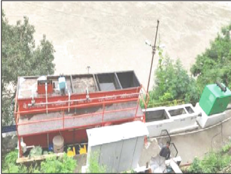
Fig. 25.2 A view of the 50 KLD STP at the site
