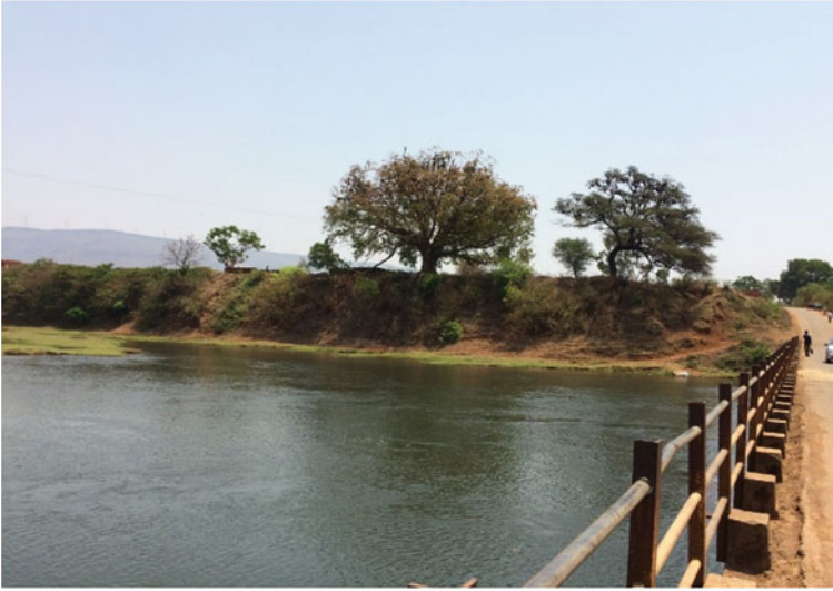
Picture 1 Erosive bank on southern side of river
