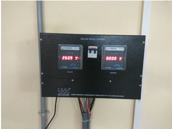
Fig. 11.5 Data logger across batteries
