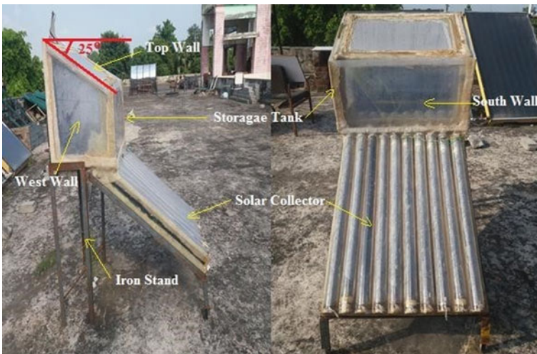
Fig. 1 Photograph of TDSWHS installed at MNNIT Allahabad
