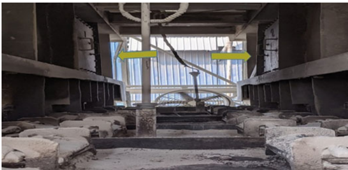
Fig. 3 Designing man-hole at the connecting channel area of D-shape twin shaft kiln
