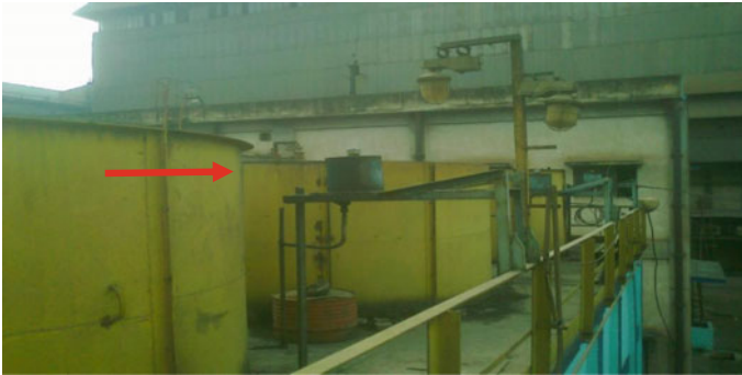
Fig. 5 Oil tank above gear box
