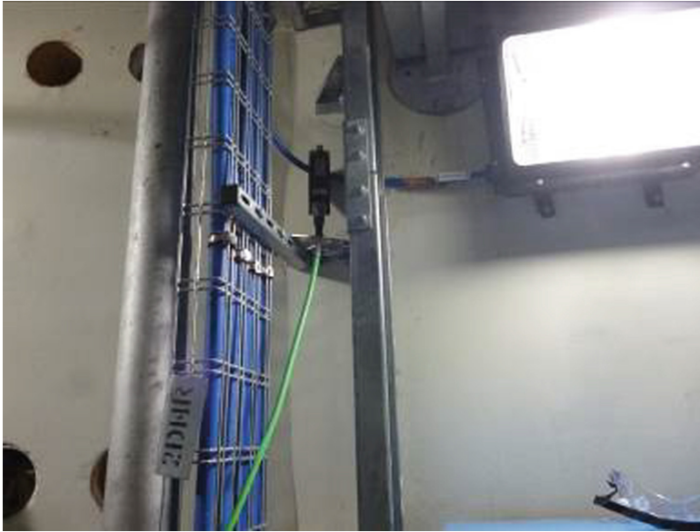
Fig. 4. Measuring the power input line of energy-saving lamp with current probe
