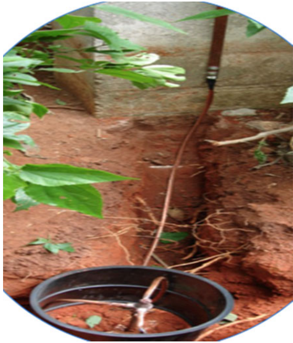
Fig. 12 Earth joint box and connections
