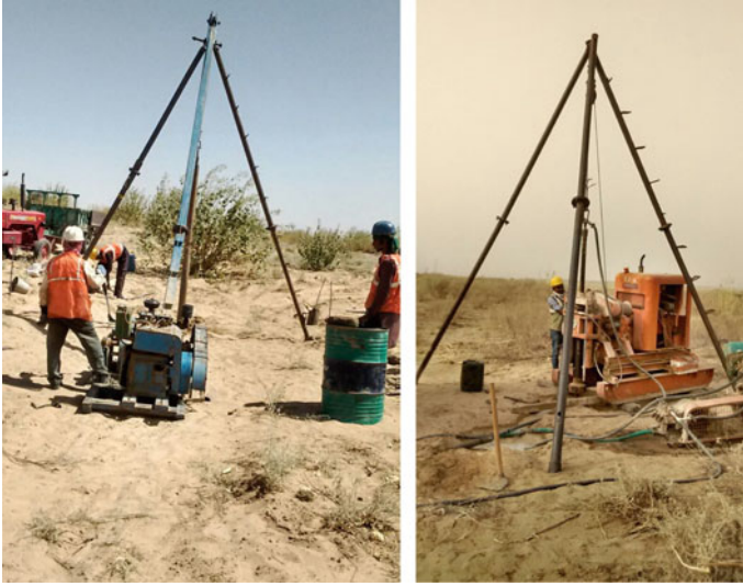
Fig. 2 Boreholes in progress. Photo on left illustrates soil boring in progress using mechanized shell and auger. Photo on right illustrates rock coring being done using hydraulic rotary rig
