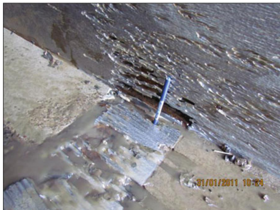
Fig. 18.9 Abrasion to a sill beam and concrete
