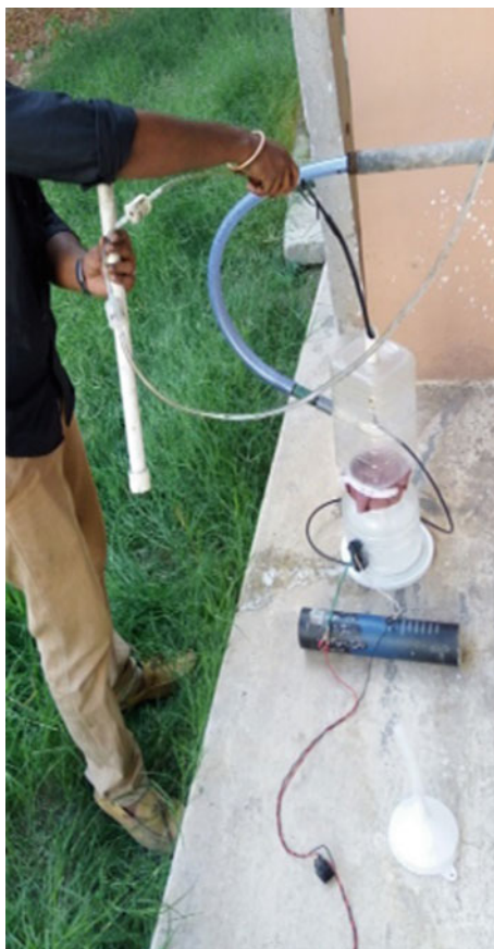
Fig. 3 Slaking calcium hydroxide solution unit with sprayer capacity of 60 L/h
