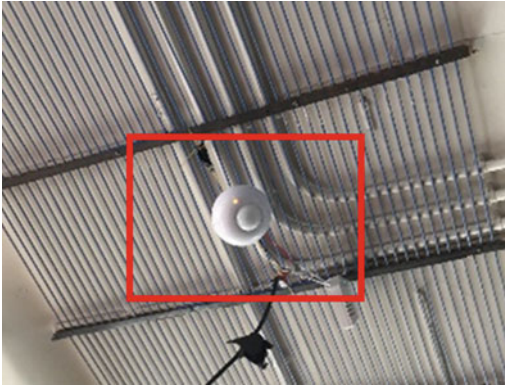
Fig. 5.10 Illustration of installed PIR sensor
