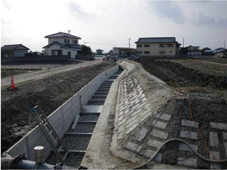
Fig. 4.3 An environment-conscious construction method allowing expansion of canal width. Gently sloping eco-blocks are used on the side of lotus root fields
