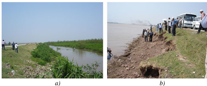
Fig. 19.5 Seadykes protected by mangroves (a) and seadyke eroded due to absence of protection mangroves (b) in Northern Vietnam (Image source: Phan Hong Anh)
