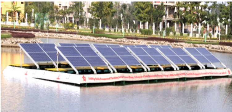
Fig. 2 10 KW FPV plant at Rajarhat in Kolkata [8]
