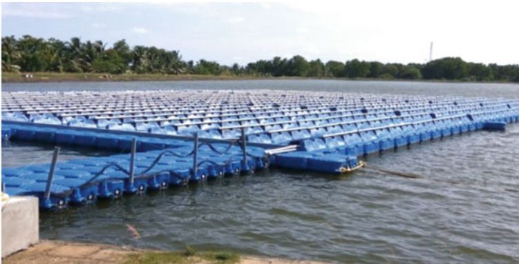
Fig. 4 100 KW FPV plant at Kayamkulam, Kerala [10]
