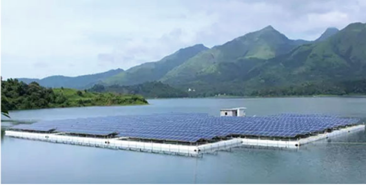
Fig. 3 500 KW FPV plant at Wayanad in Kerala [9]
