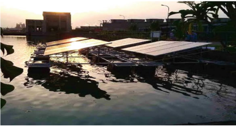
Fig. 8 4.8 KW FPV plant in Nagpur [14]
