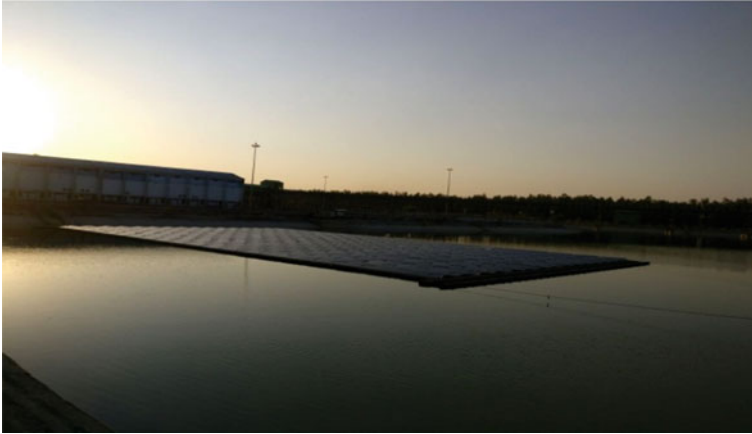
Fig. 9 100 KW FPV plant at Panipat in Haryana [11]
