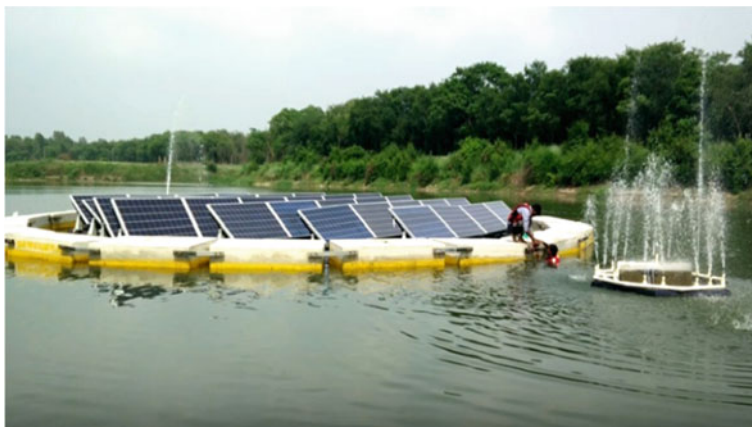
Fig. 5 10 KW FPV plant in Chandigarh [11]
