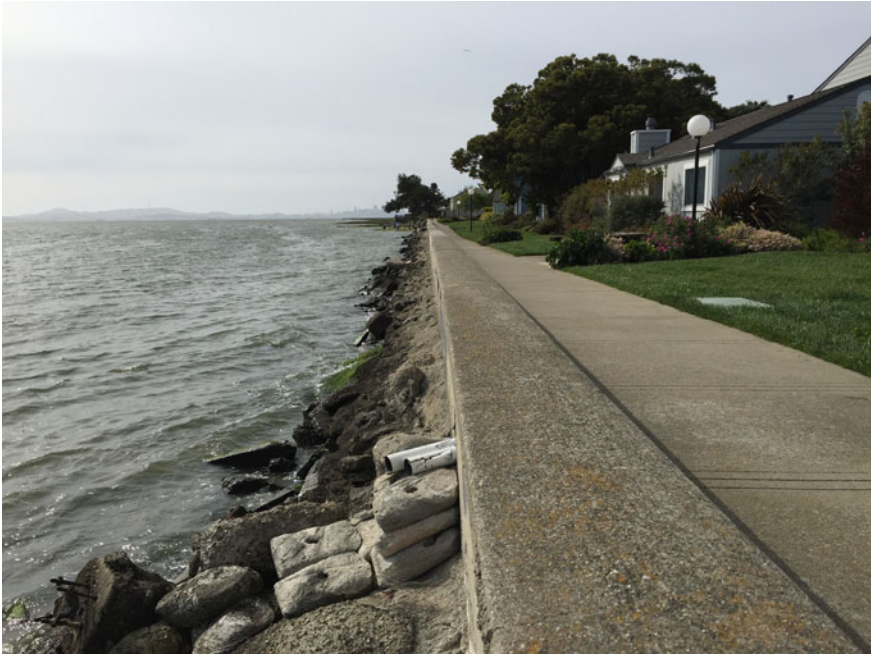
Fig. 4 Existing seawall along the coast of the City of Alameda, California, on San Francisco Bay (photocredit: K. Hill)
