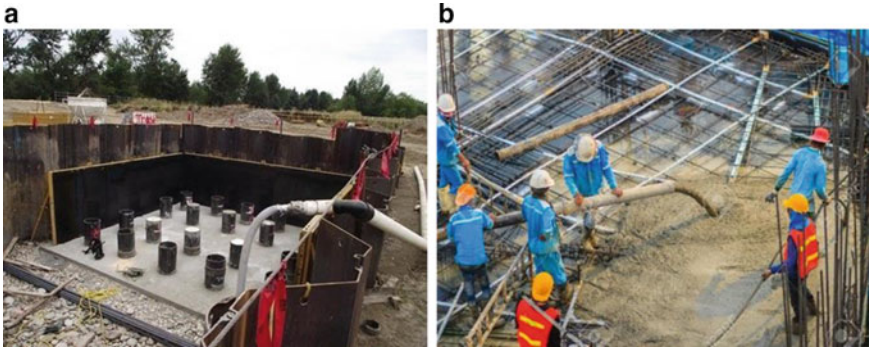
Fig. 1 a) Bottom layer of the floor b) Concrete blinding of the floor
