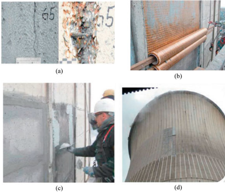
Fig. 21 Strengthening of cooling tower, Germany. a Damage extent; b strengthening using PBO-FRCM; c surface finishing and d final view (Picture Courtesy Ruredil SPA)
