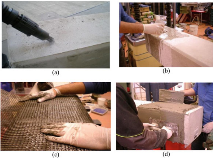
Fig. 7 Strengthening using FRCM system. a Surface preparation; b surface wetting; c FRCM application and d finishing (Picture Courtesy Escrig et al. 2015)
