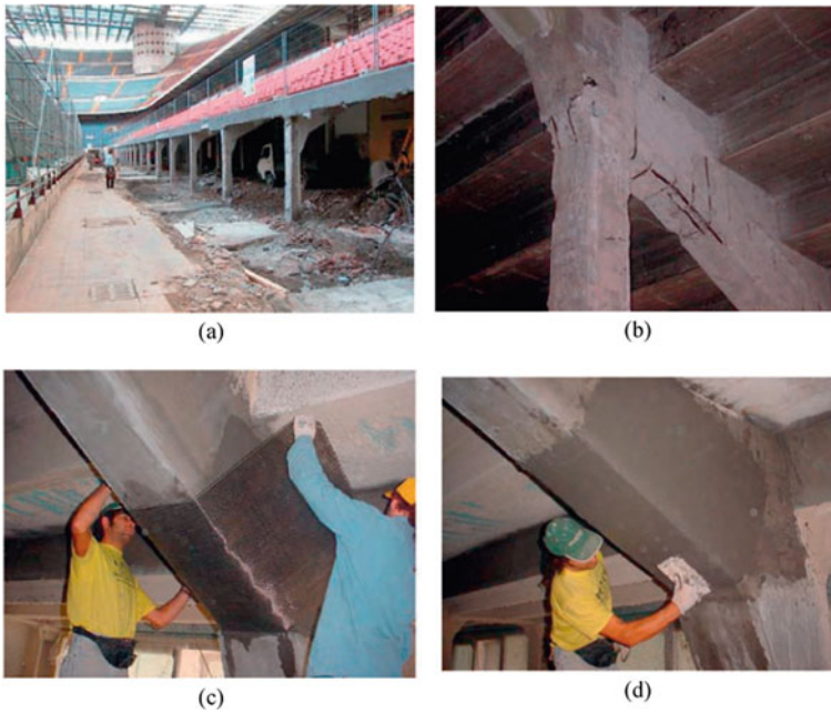
Fig. 20 Strengthening San Siro stadium. a Site view; b preliminary assessment; c strengthening by U-shaped FRCM and d surface finishing with cementitious grout (Picture Courtesy Trimboli and Mantegazza 2004)
