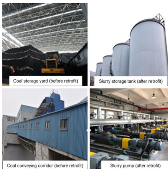
Fig. 44.4 Comparison of heat plant environment before and after the retrofit
