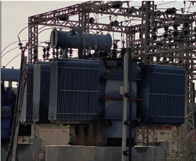
Fig. 1 5-MVA stadium transformer
