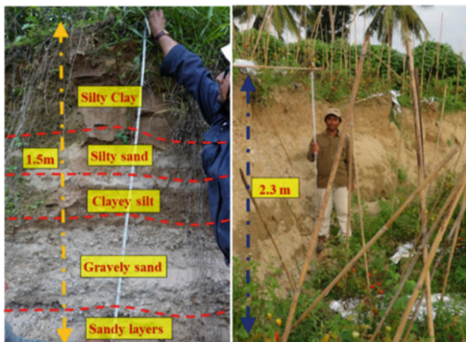
Fig. 12.14 Profile of exposed soil layer due to the extensional cracks near PDCPT1 (Hazarika et al. 2020)
