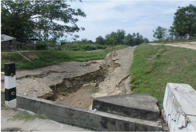
Fig. 12.29 Damage to the embankment of irrigation channel (Kiyota et al. 2020)
