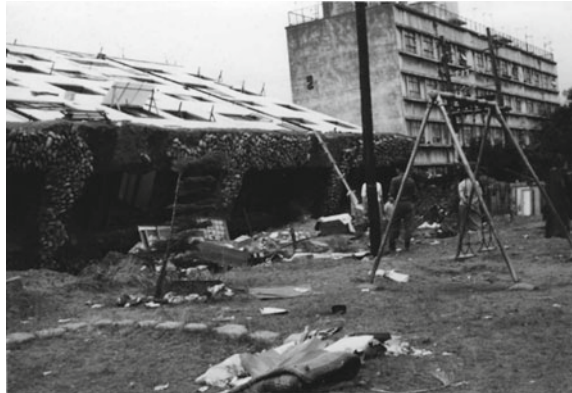
Fig. 3.1 Tilting of apartment building in Kawagishi-cho site of Niigata (by reconnaissance team, department of Civil Engg, Univ. Tokyo)
