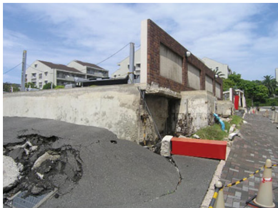
Fig. 3.2 Floating of underground parking lot in Yokohama City in 2011
