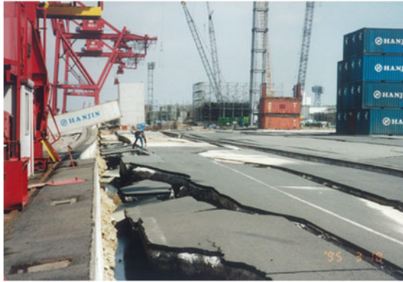
Fig. 3.3 Liquefaction-induced lateral displacement of quay wall in Kobe Harbor
