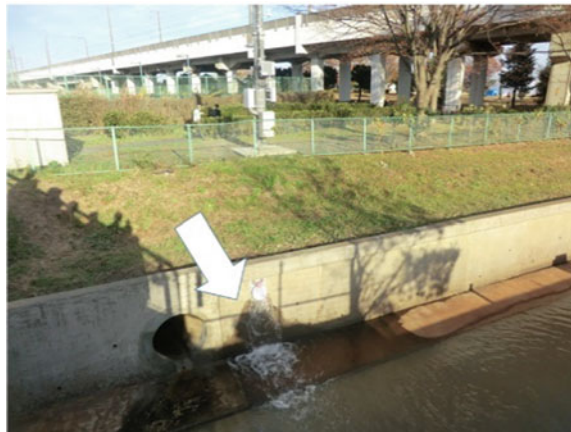
Fig. 3.43 Drainage of water from Kuki City (photo by Prof. J. Koseki)
