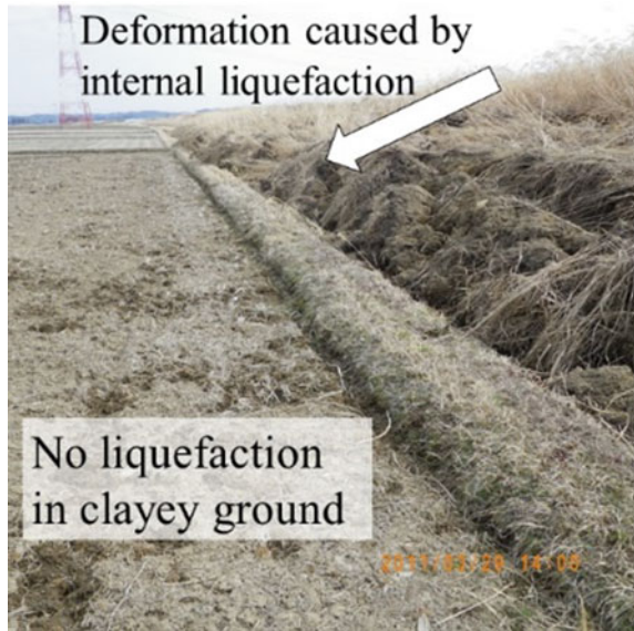
Fig. 3.39 Deformation of levee resting on vulnerable soil induced by internal liquefaction (Naruse River during the 2011 Tohoku earthquake)
