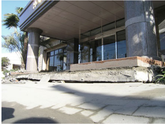
Fig. 3.33 Differential settlement between pile-supported building and surrounding liquefied ground (in Urayasu 2011)
