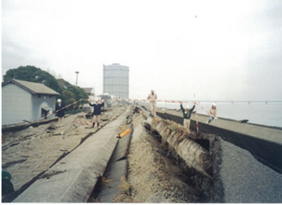
Fig. 3.36 Liquefaction-induced subsidence of Yodo River levee
