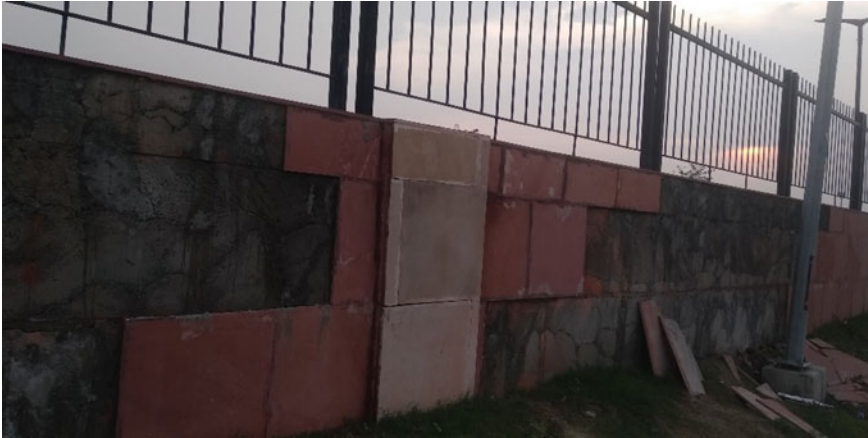
Fig. 8 Condition of tiles on wall in early stages of construction near Bambala Puliya, Tonk road
