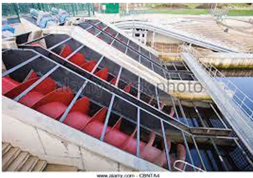
Fig. 4 Screw hydro turbine multiple installation
