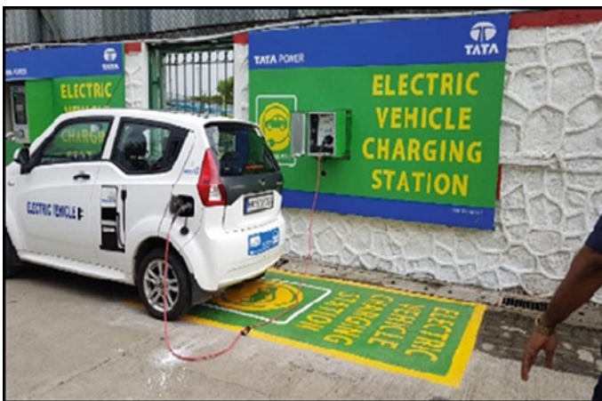
Fig. 7 EV charging station at Vikhroli, Mumbai (owned, operated and managed by Tata Power)
