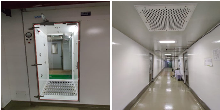
Fig. 26.3 Airlock and HVAC for SPF rooms entry
