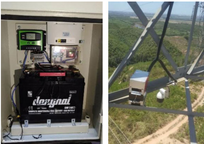
Fig. 4 IoT station box on high voltage transmission line tower
