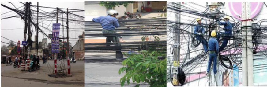
Fig. 3 Images of overhead lines—a mess for repair or replacement [9]
