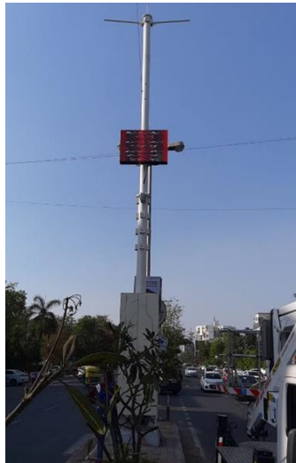
Fig. 4. Modular infrastructure installed in the city
