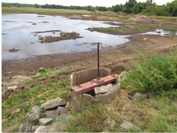
Fig. 15.2 Typical degraded small tank in a cascade. Photo credit Shamen Vidanage
