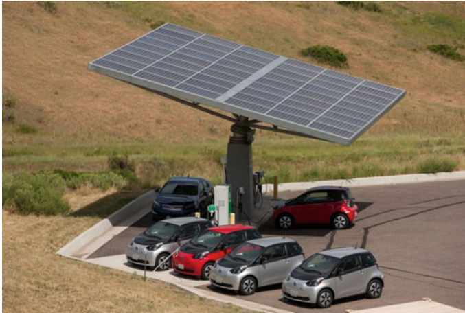
Fig. 5 Solar-based EV charging station (Mouli et al. 2015)
