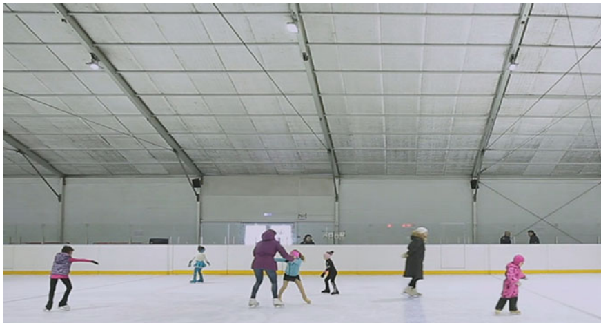
Fig. 14 Insulating coating of ice skating rink (owned by our company)
