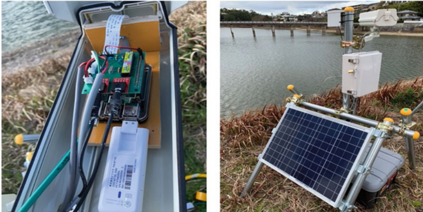
Fig. 7.7 Installed devices and solar panel for the Kaerumata Reservoir
