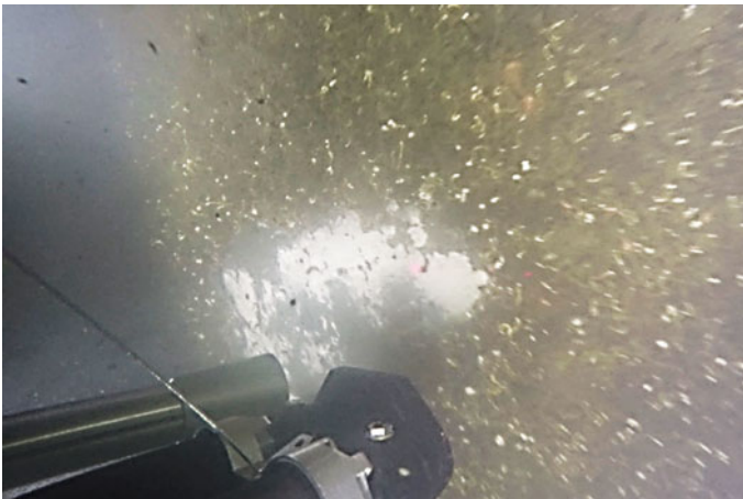
Fig. 9 Snapshot taken during the removal of marine growth from the piles using high-pressure water jets; the cleaned area appears brighter in the photograph as a result of marine growth removal
