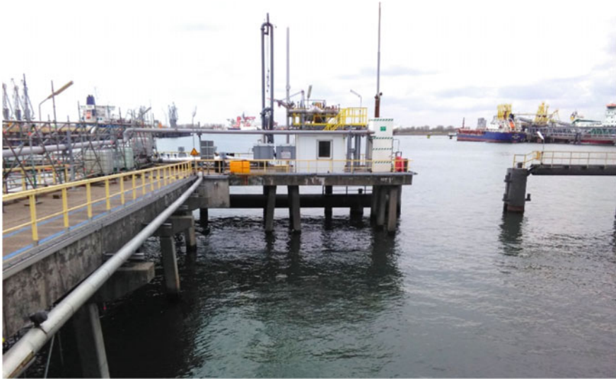
Fig. 7 Photograph of the part of the jetty showing the steel piles to be inspected
