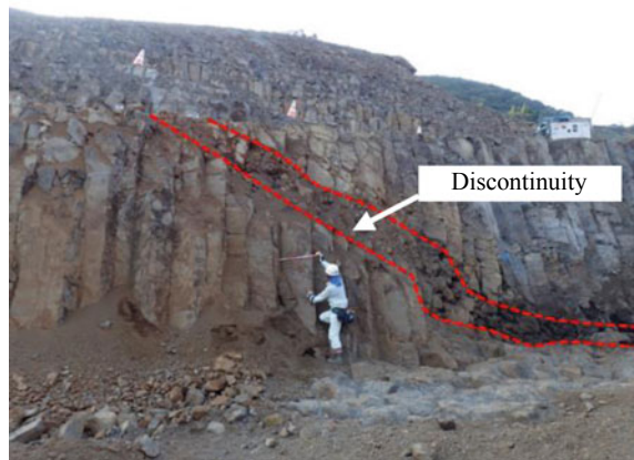
Fig. 3 Discontinuity observed at cut slope of right bank
