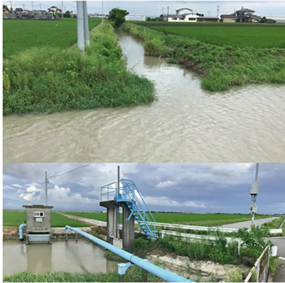
Fig. 4 Storage gate and pump for pumping installed in the irrigation channel “Creek”
