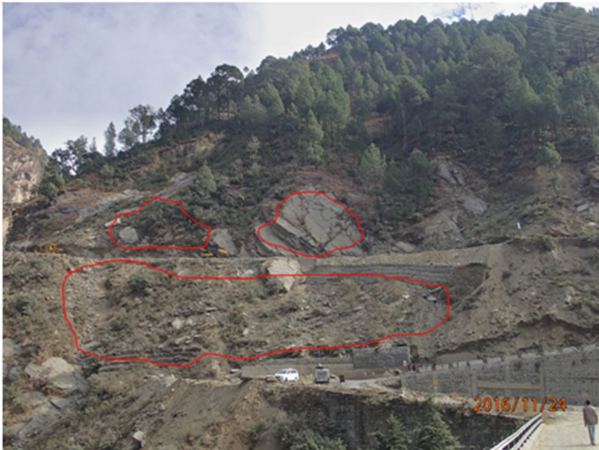
Fig. 1 Two-slided portions with hill side and valley side unstable patches at Birahi
