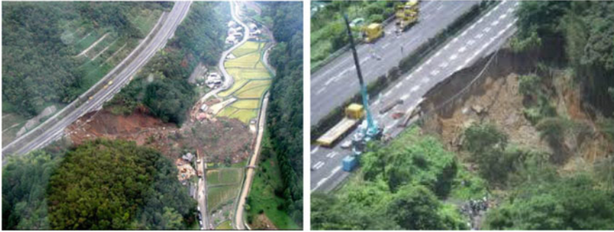
Photo 1 Road embankment failure due to heavy rain [1] and large earthquake [2]
