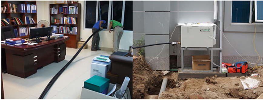
Fig. 10 GSHP installation at VIGMR, Hanoi, Vietnam
