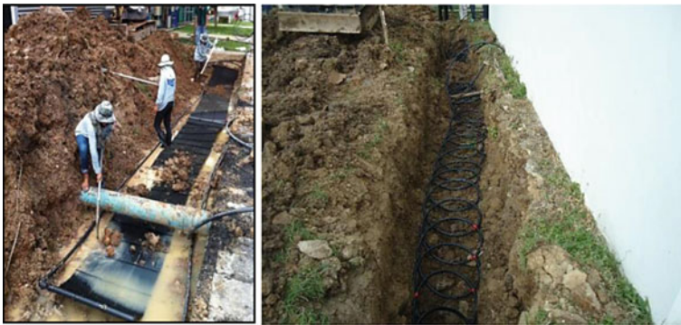
Fig. 6 Installation of capillary mat heat exchanger (left) and slinky-configured HDPE pipe (right)
