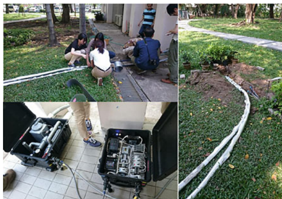
Fig. 13 TRT measurement at the GSHP site at Chulalongkorn University, Bangkok Campus
