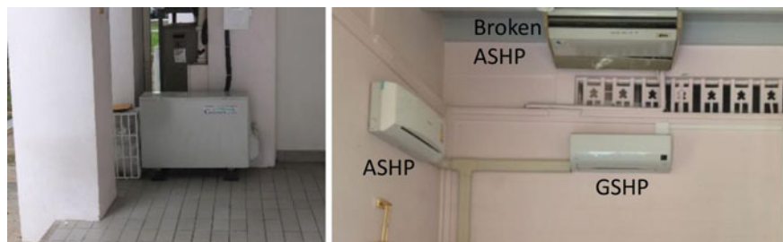
Fig. 5 Heat pump (left) and fan coil units (right). ASHP was installed for performance comparison analysis at Chulalongkorn University, Bangkok
