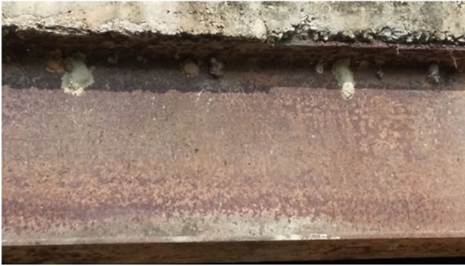
Fig. 1 Typical corrosions on steel beam structure
