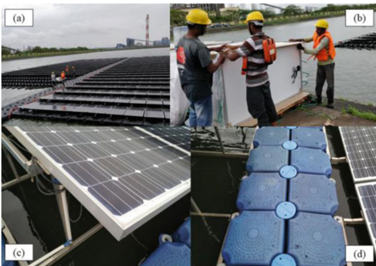
Fig. 21.4 a A multitude of ergonomic hazards during installation; b work near water exposes the workers to a combination of hazards; c sharp edges and presence of electricity are occupational hazards, and; d work on unstable floaters presents additional hazards
