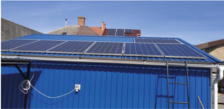
Fig. 5. Measured solar panels on the roof of a garage.
