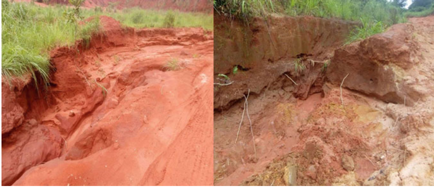
Plate 16.3 Showed the condition of adjoining farmlands that have been abandoned due to high levels of flooding during the wet seasons. This has affected agricultural production along the Odor River and led to land fragmentation
