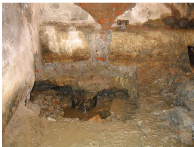
Fig. 5 Photo of wood sills and wooden piles under the foundation of five-floor building
