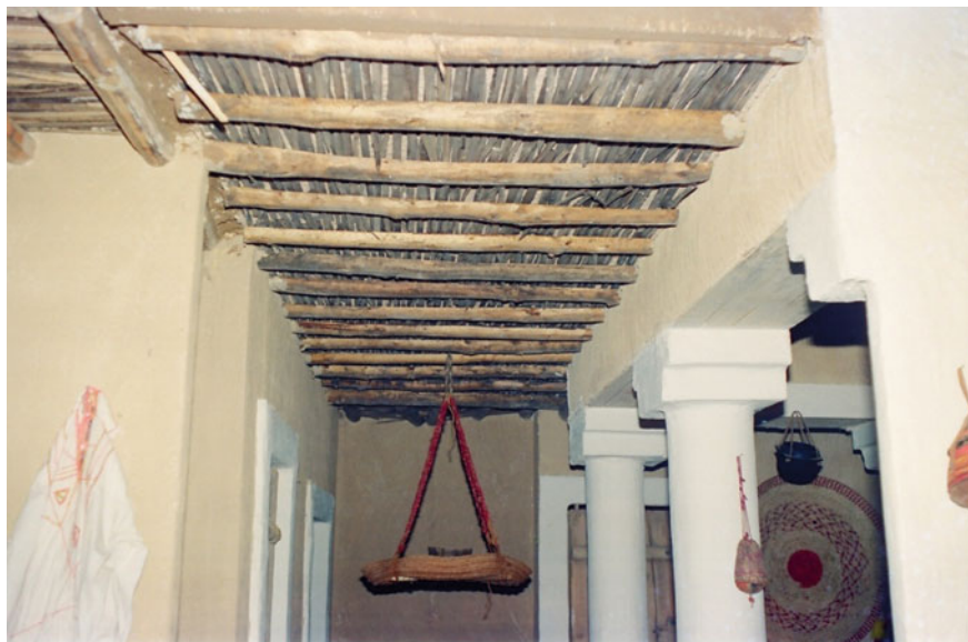
Fig. 30 Roofing using palm midribs over a series of tree branches as beams, Fayoum, Egypt
