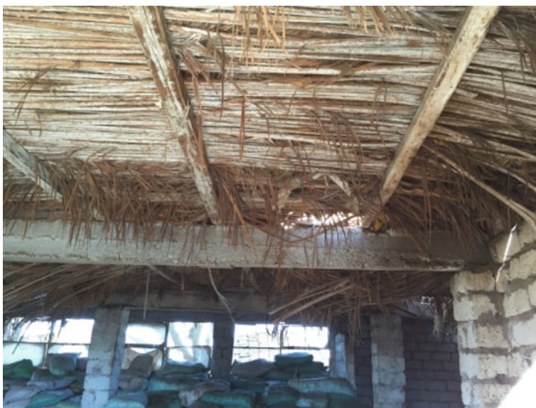
Fig. 24 Date palm leaves over wooden poles for roofing in a storage house in Menya, Egypt
