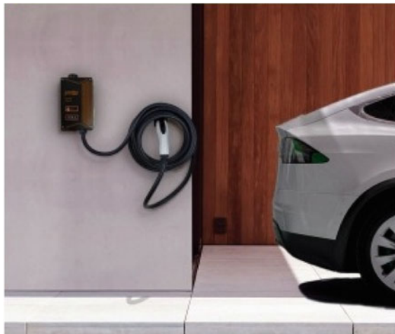
Fig. 17 Level one charging [11]. Source New Car Kids
