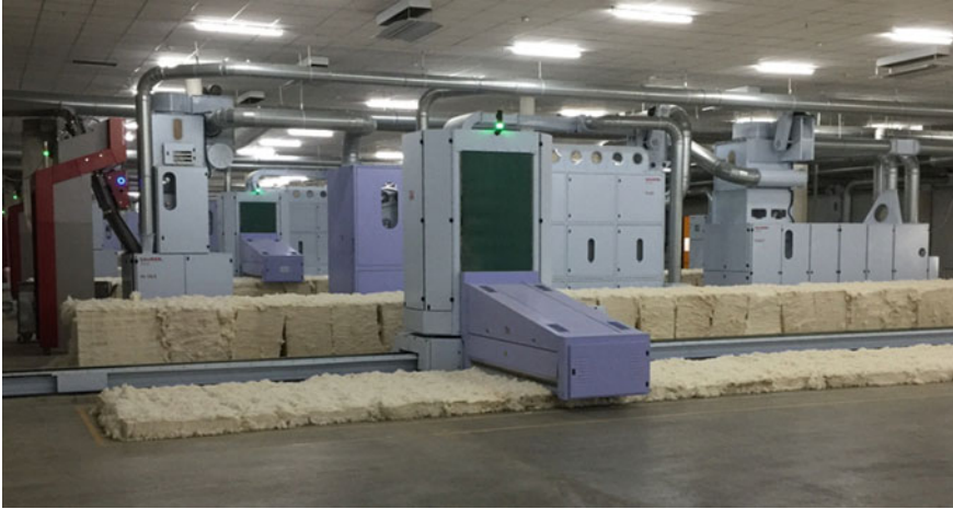
Fig. 8.1 Automatic bale opener installed in the cotton spinning industry in Uzbekistan
