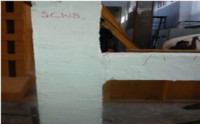
Fig. 5 Cracking pattern of beam–column joint SCWB
