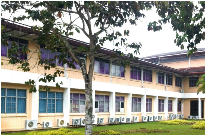
Fig. 2 Photograph of floor-mounted outdoor units that are part of air-cooled split unit air-conditioners
